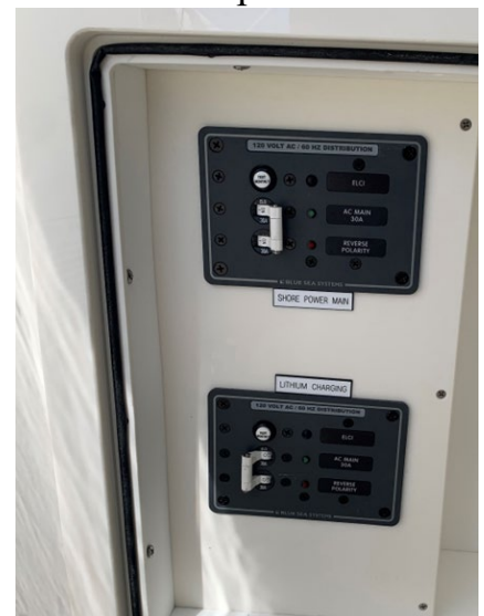
Port Cockpit cabinet
