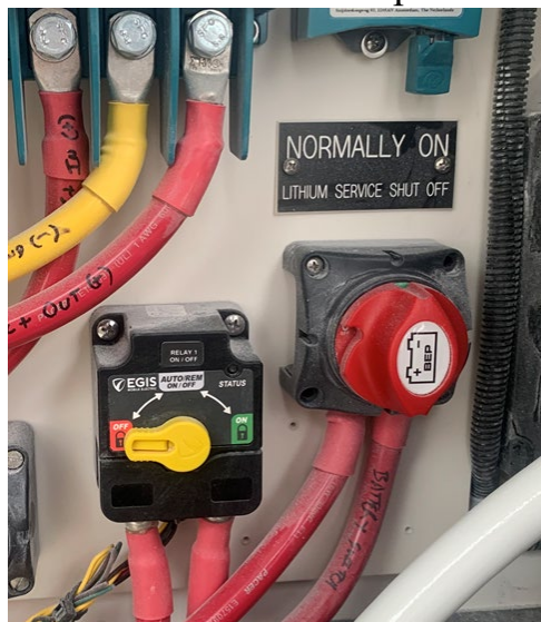
Stbd Aft Mech Space
