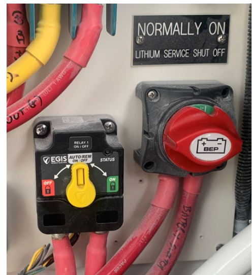
Stbd Aft Mech Space
