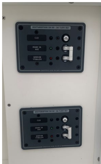
Port Cockpit cabinet
