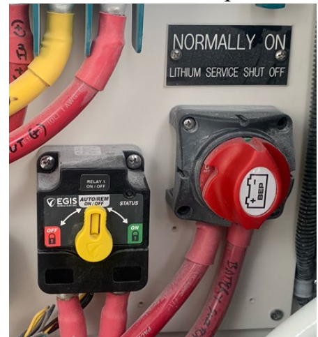
Stbd Aft Mech Space
